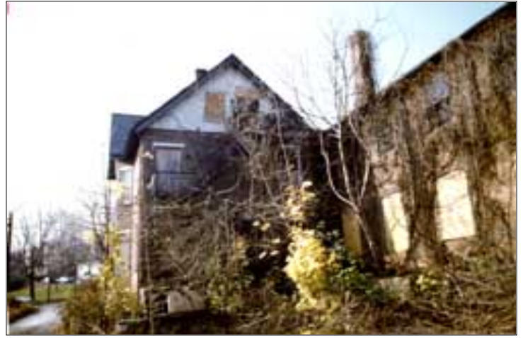
Boarding up without adequate ventilation and maintenance has accelerated deterioration of this property. Photo: NPS files.
