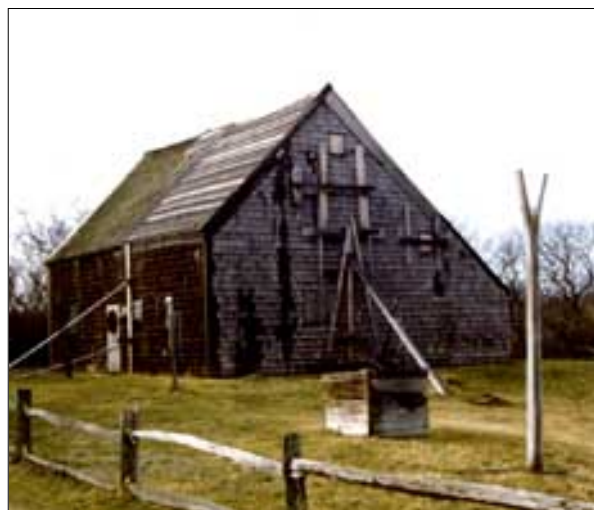
Buildings seriously damaged by storms or deterioration may need to be braced before architectural evaluations can be made. Photo: John Milner Architects. Photo: NPS files
