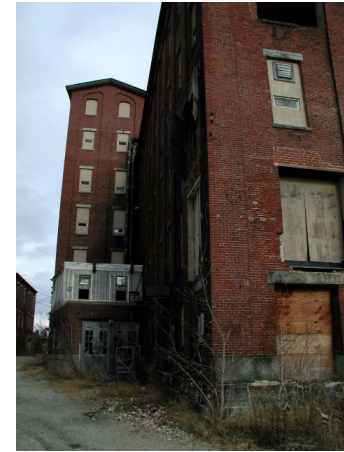
Owner: Absentee or Unknown Building Deteriorating Open to Unauthorized Entry
