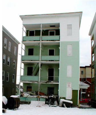
Owner: Unresponsive Uninhabited Open to Unauthorized Entry
